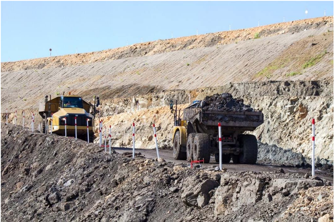
Figure 1: Articulated dump trucks exiting and entering the Siana open pit via the primary ramp
