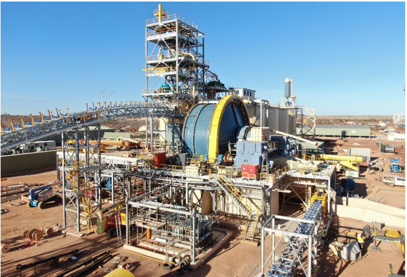
Figure 2: SAG mill shell, motors, girth gear, mill lubrication skid and process plant control room are now in position.
