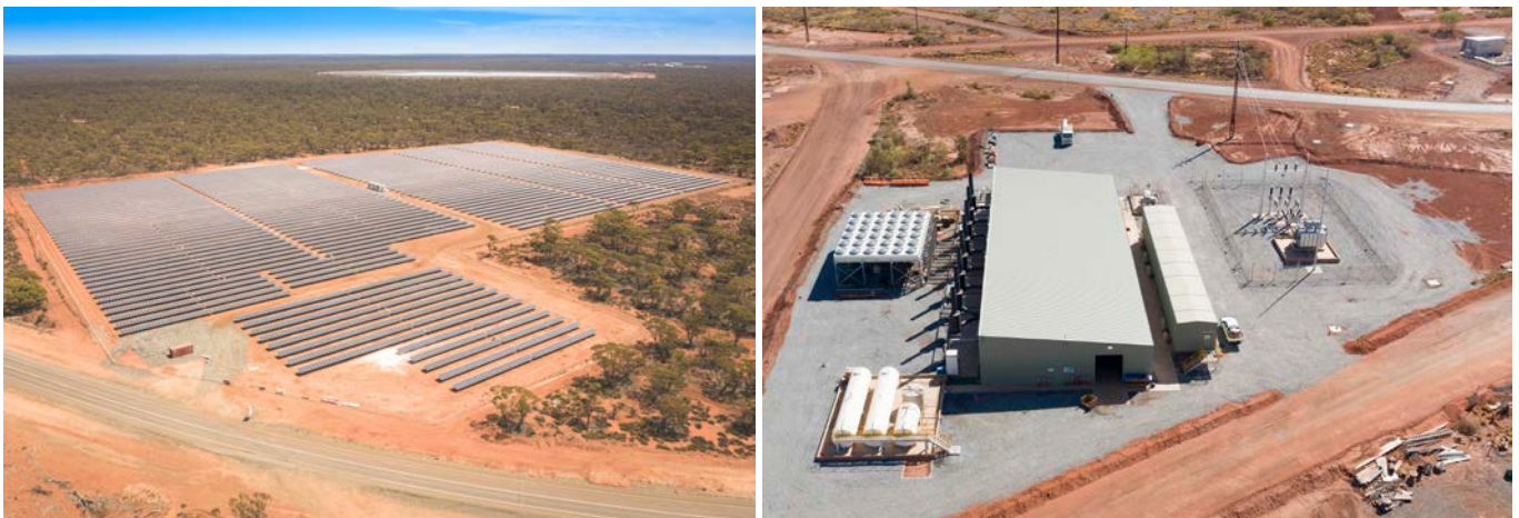
Figure 1: Zenith power installations similar to that which will be built and operated at KOTH.
