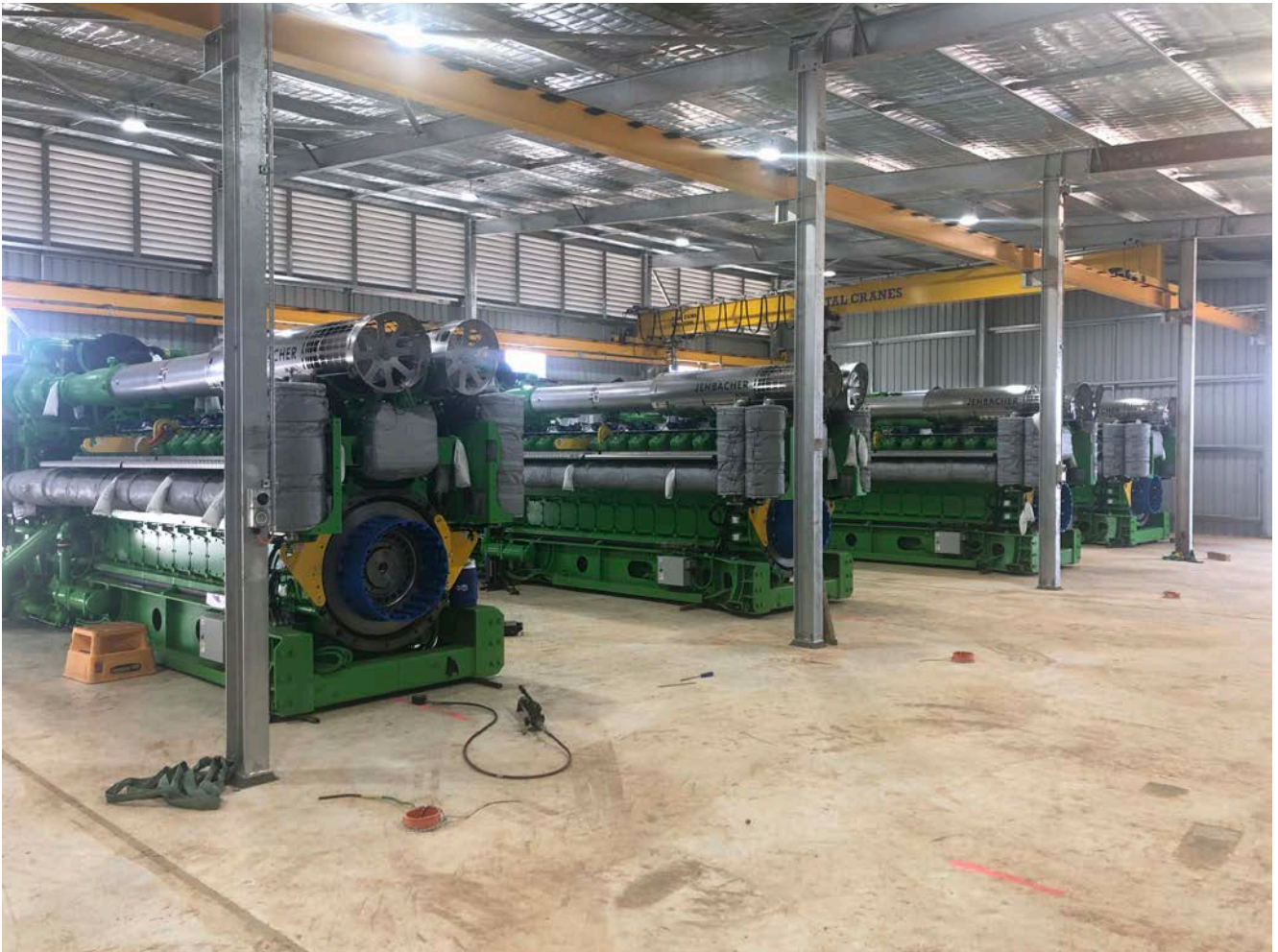
Figure 3: Delivery and installation of the Jenbacher gas turbine engines as at 6 December (pictured within Zenith’s power station building).
