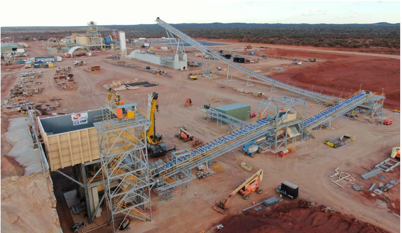
Figure 1: The gyratory crusher is now installed, with the crushed ore stockpile reclaim area and process plant in the background.
