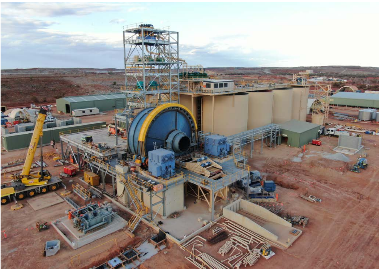
Figure 2: SAG mill shell, motors, girth gear, mill lubrication skid and process plant control room now in position.
