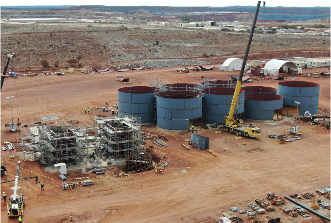
Figure 2: Preparation for the concrete pour of the plinths for the processing plant is underway.
