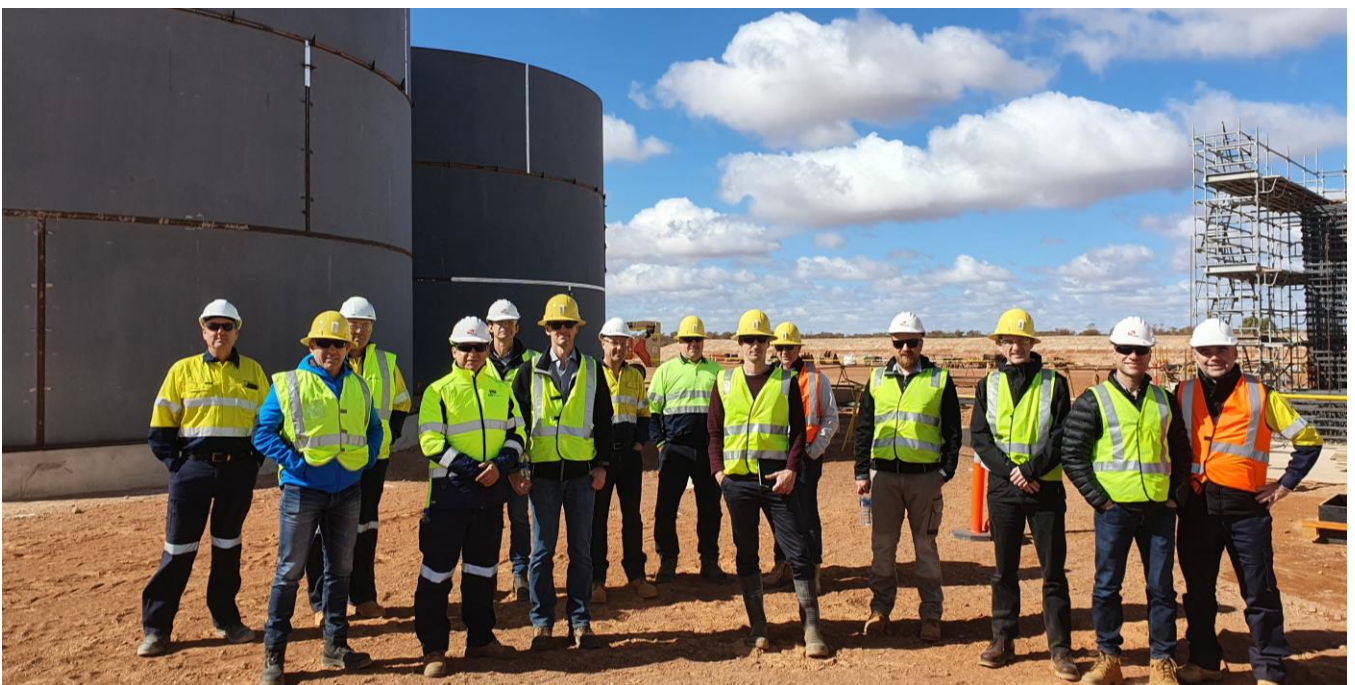
Figure 5: The Syndicate Banks visited KOTH on 24 May 2021 to see construction progress on site.
