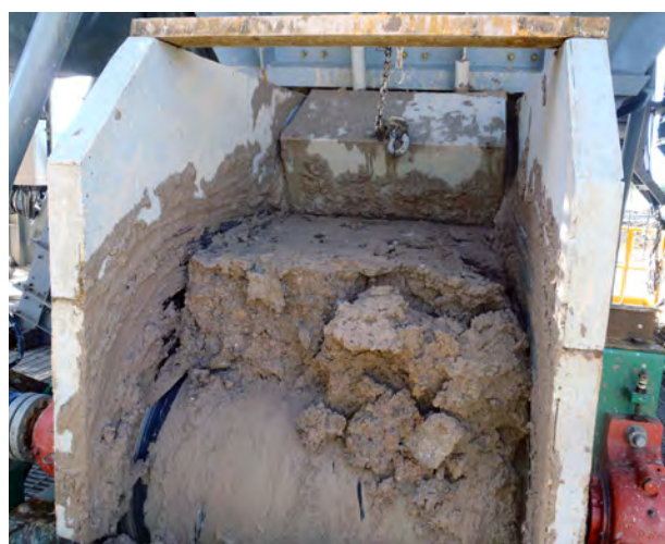
SAG Mill conveyor feeder
