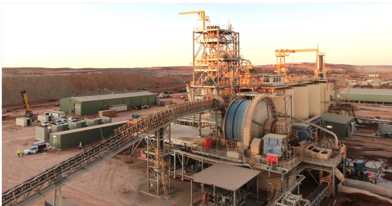
Figure 1: The new KOTH processing plant achieved its first gold pour milestone on 5 June 2022.
