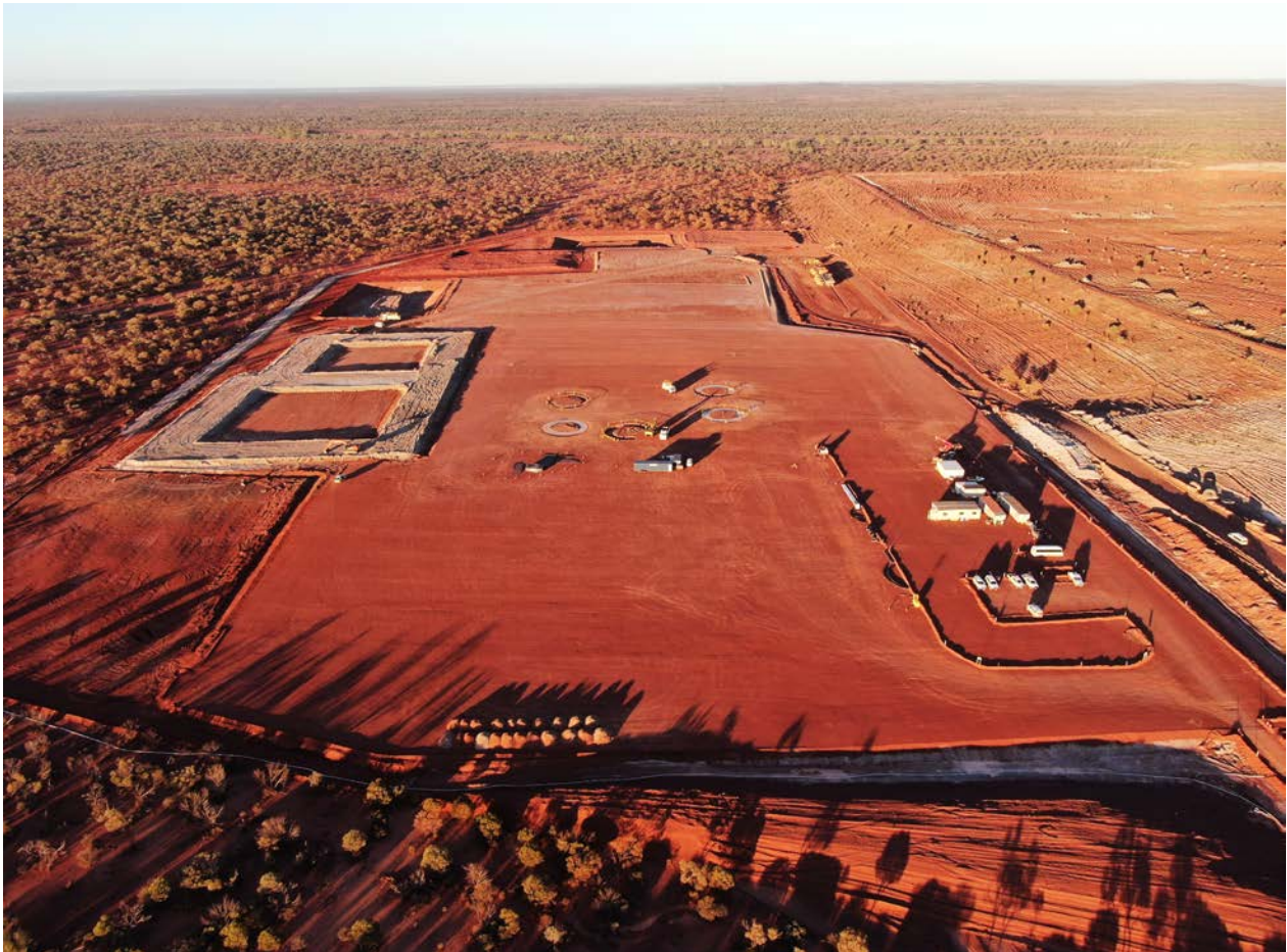
Figure 1: Current site of the future KOTH mill, with bulk earthworks sufficiently progressed to allow the concrete contractor to commence. Construction of CIL tank foundations have started, and the Raw and Process Water Ponds earthworks are in progress.
