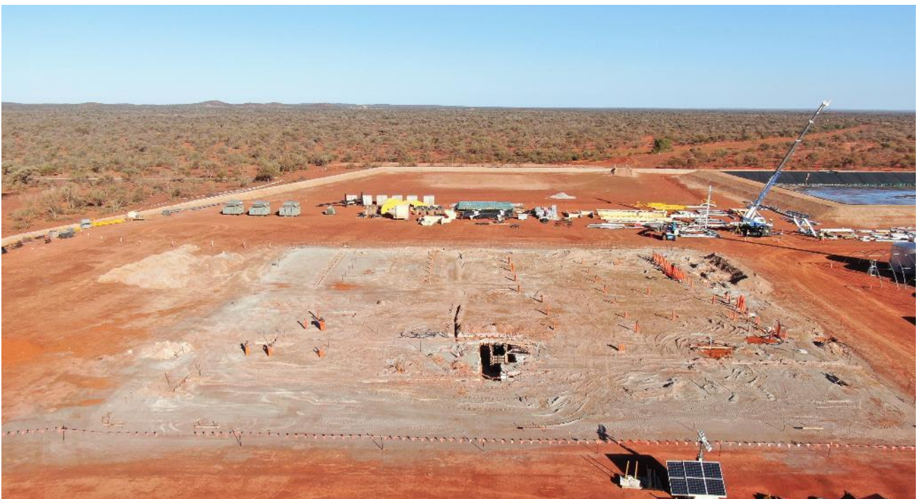
Figure 3: Power station site at 3 August 2021 – trenching, conduit installation, and switchroom/generator hall footings have commenced.
