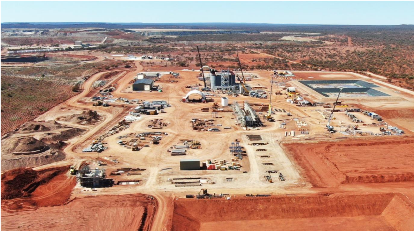
Figure 2: Construction progress at 7 August 2021 – crusher in the foreground, stockpile reclaim tunnel in the centre, mill and CIL tanks at the rear of the photo.
