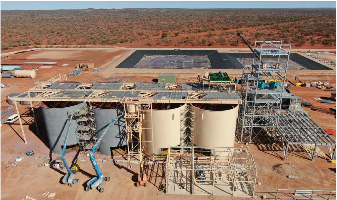
Figure 3: Elution column is now installed and erection of the gold room steelwork is underway.
