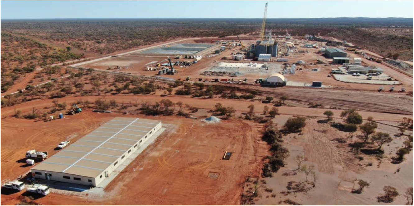
Figure 4: The mine services building is fully assembled, and the fit-out is ongoing.
