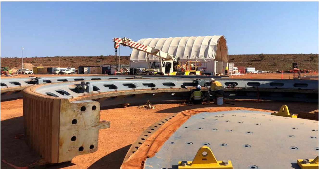
Figure 3: Assembly of the girth gear for the 36-foot diameter SAG Mill being assembled on site.
