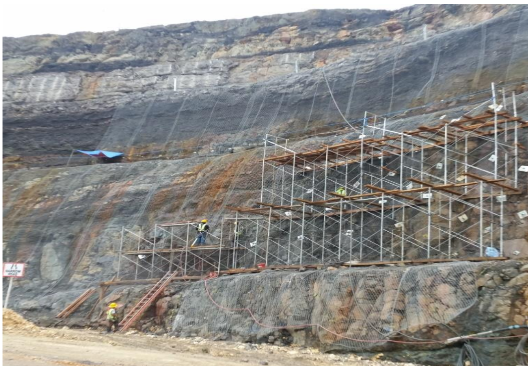
Figure 1: Installed rock bolts and wire mesh ahead of shotcreting at the -22m RL portal, Siana Underground Development
